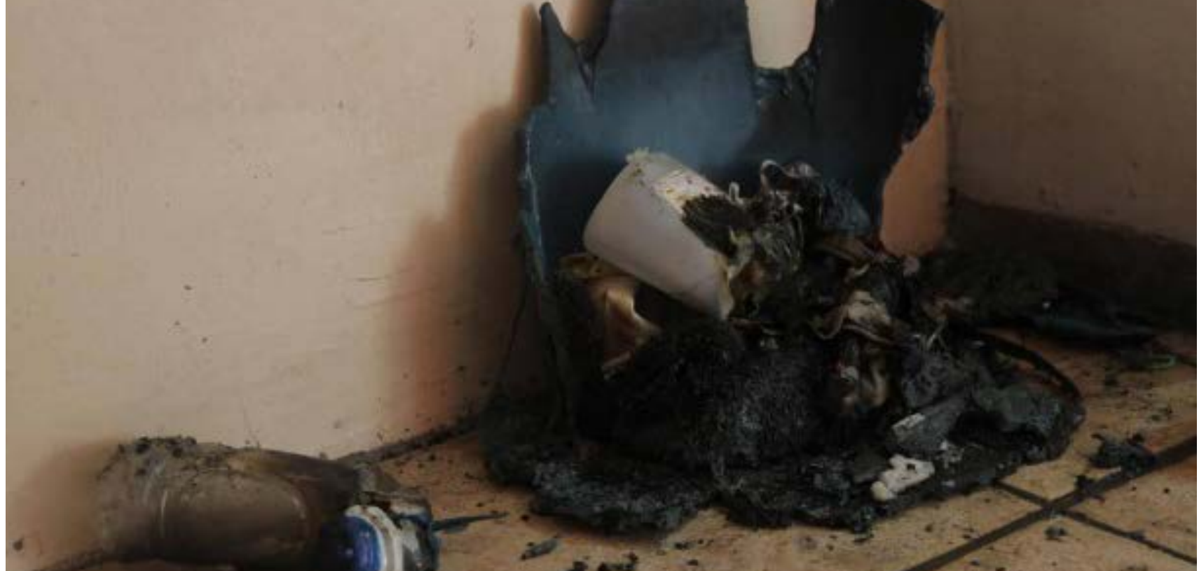
A burnt trash bin placed outside the male restroom in the fifth floor Finster building serves as an evidence of the arson incidents. Photo/ Reil Benedict Obinque
